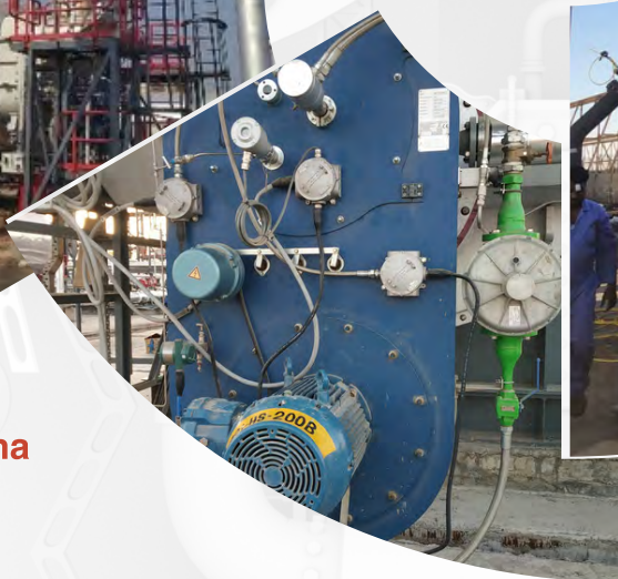
Heater Treater Mehsana field, ONGC (India)
